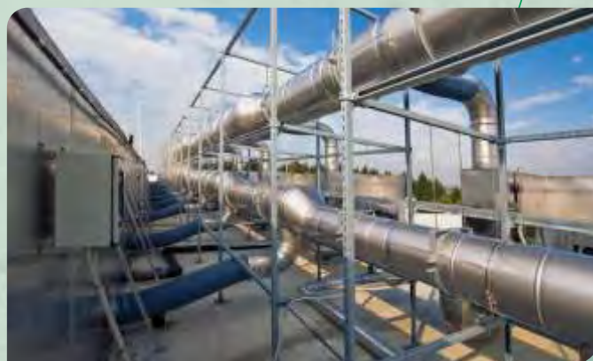
Ventilation system at Composting plant
