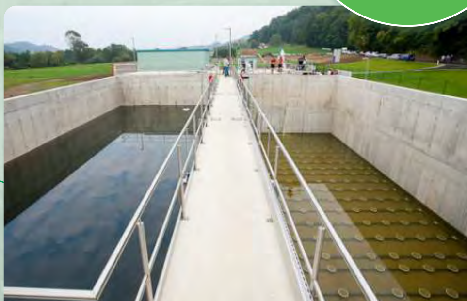
Central waste water treatment plant Šentjur
